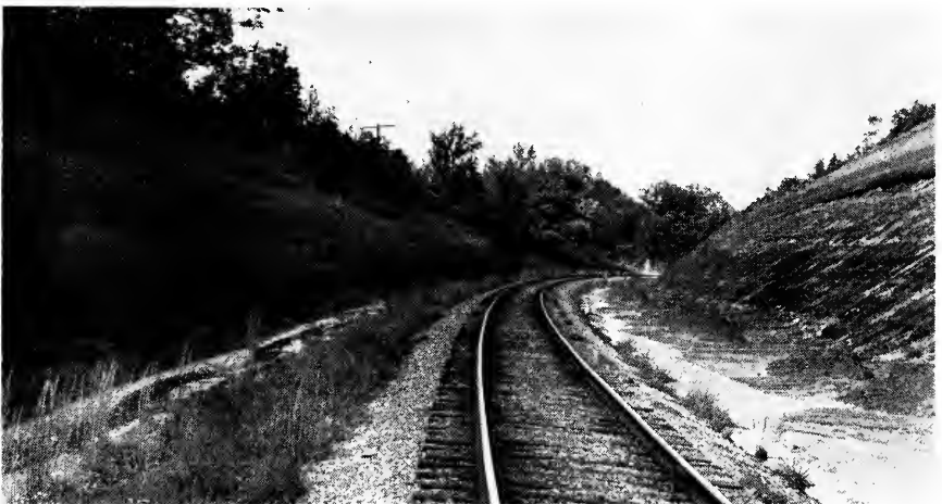
Fig. 2— 1\frac{1}{2} :1 cut slopes in sandy clay and soft shale.
